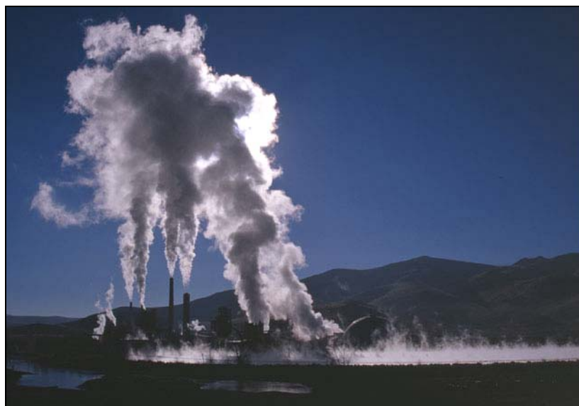
Steam plumes rising from cooling towers, boiler stacks, and cooling pond at Tracy Generating Station east of Sparks. Huge volumes of water are used to operate steam electric power plants. New power plants using air-cooled and hybrid-cooling towers can reduce cooling water use by 98%, conserving the state’s limited water and protecting aquatic ecosystems. Photo © Mark Savage 2000.
